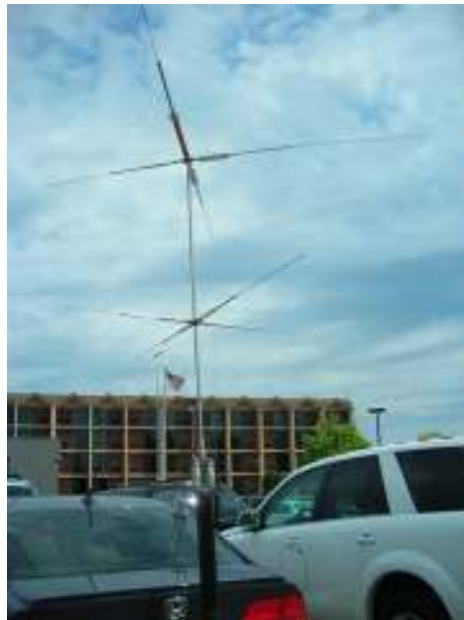
W0NAC Antenna System
